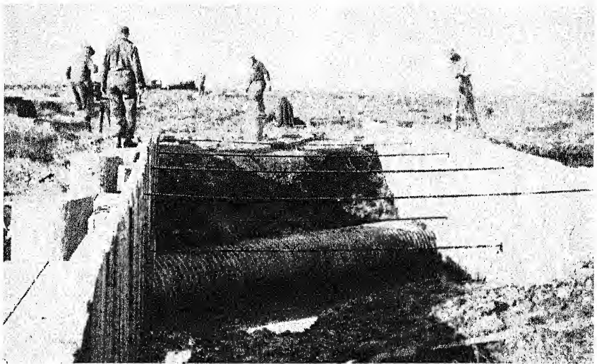
Figure 44. Corrugated metal culvert (thirty-six inch diameter) being constructed within wooden bulkheads, before being filled with earth
